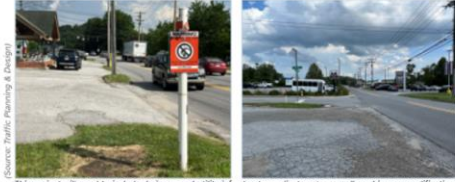
This project will need to include drainage and utility infrastructure adjustments, as well as driveway modifications and new ADA ramps.
