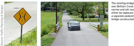
The existing bridge over Brittain Creek is narrow and will need to either be replaced or a separate pedestrian bridge constructed.
