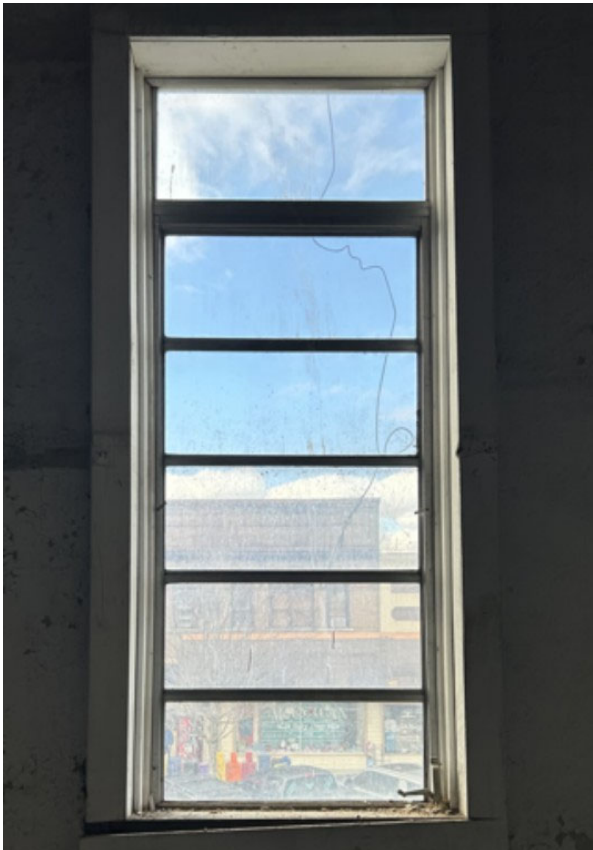
Applicant provided imagery of damaged windows
