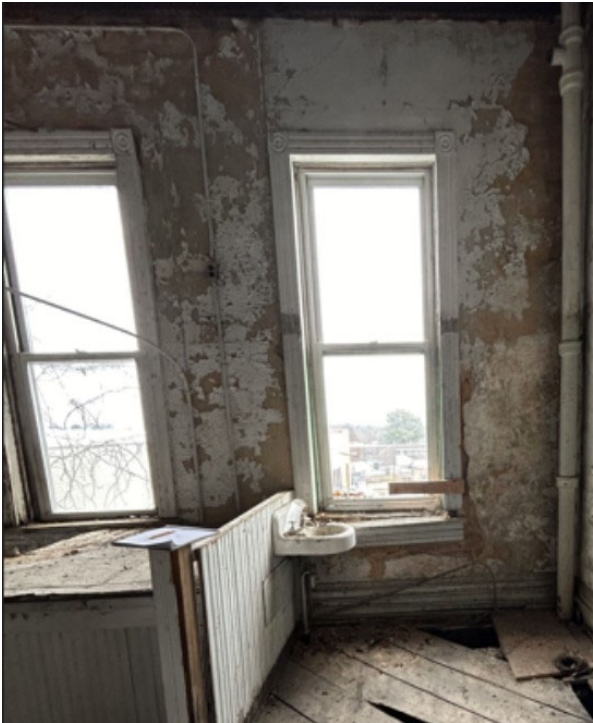
Applicant provided imagery of damaged windows
