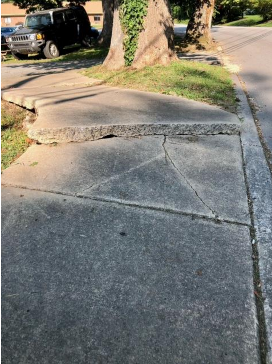
An “uprooted” sidewalk on Hebron Road at the Blue Ridge Health and Rehab Center. Simply a safety hazard for any pedestrian, handicapped or not.
