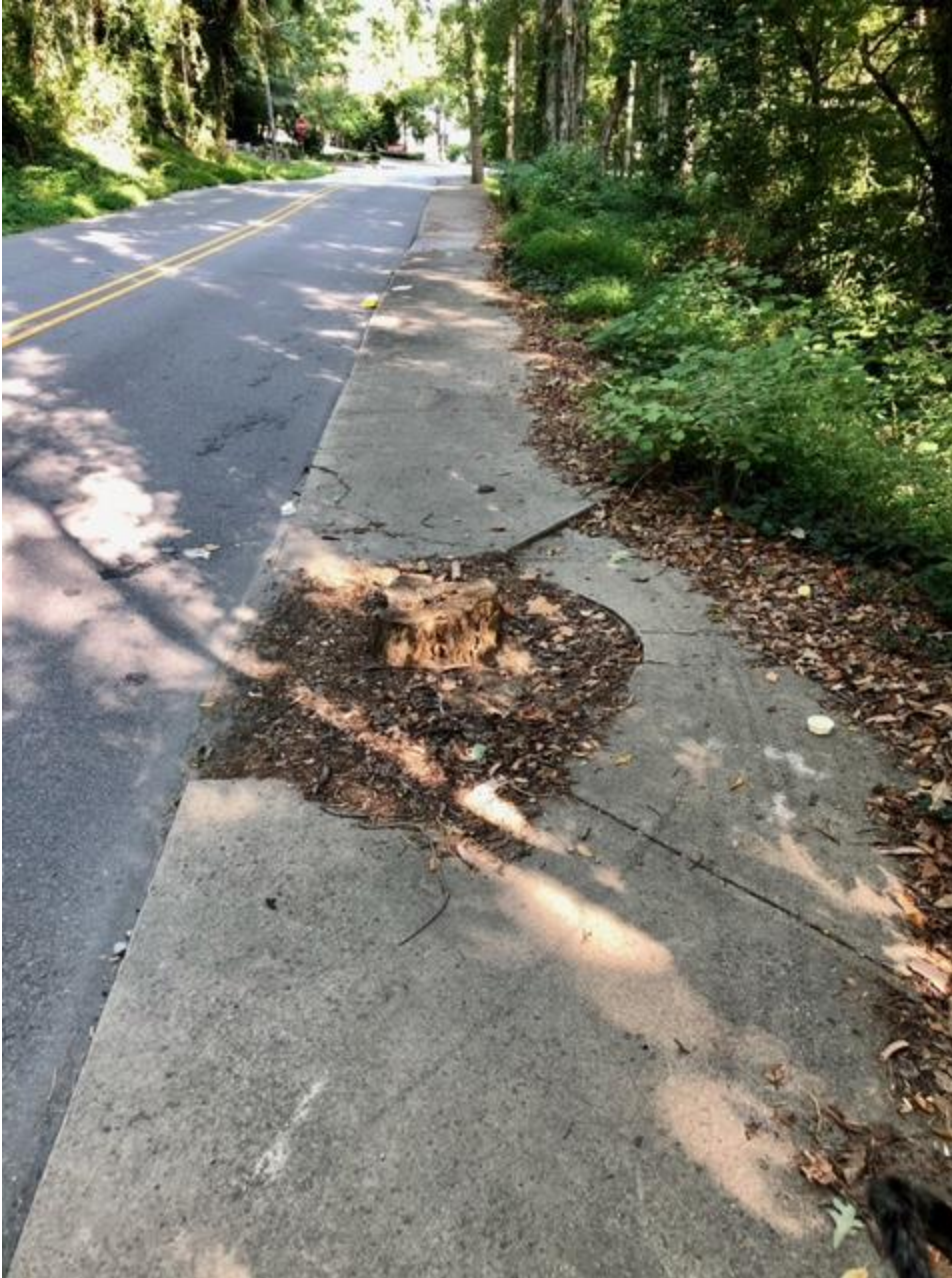
A tree stump taking up the sidewalk on West Lake Ave approaching Third Ave West. Just an obstacle for usage of wheelchairs and scooters, not to mention an eye sore.
