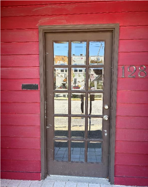
Non-original front door.
