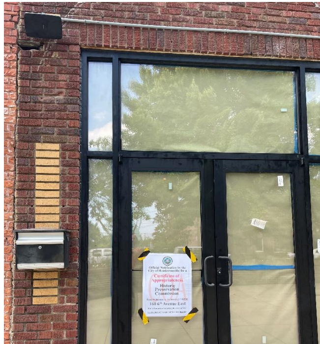
Close up view of the newly installed doors. The doors are constructed using black metal and fit into the existing storefront opening.
