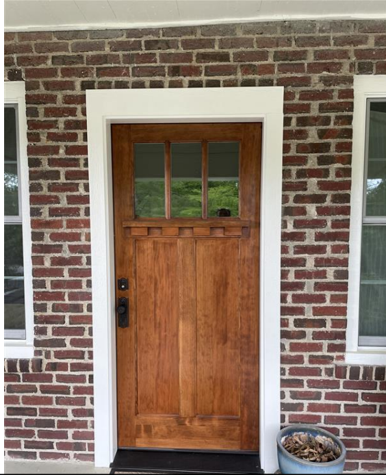
Replacement front door. Photo provided by Staff.
