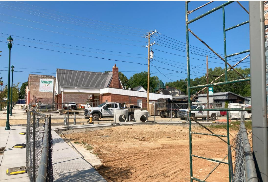
View of corner of 7 th Ave and Locust St - empty lot where existing building was recently demolished.
