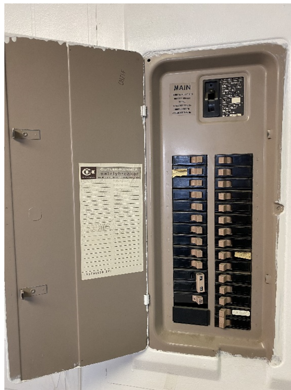
Figure 4: Existing electrical panels, appear older - need to confirm capacity for new use
