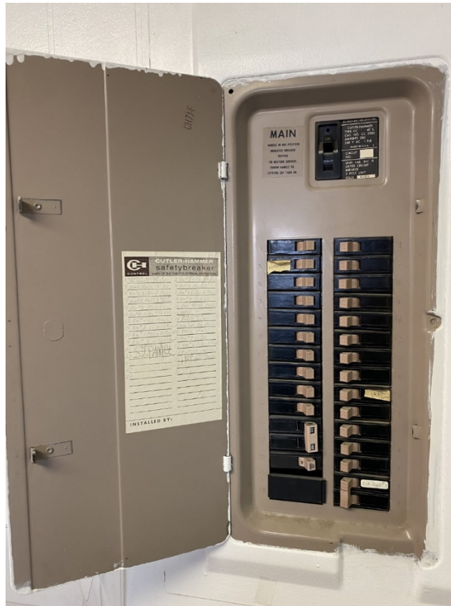
Figure 4: Existing electrical panels, appear older - need to confirm capacity for new use
