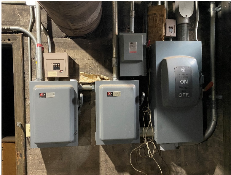
Figure 3: Existing electrical panels, appear older - need to confirm capacity for new use
