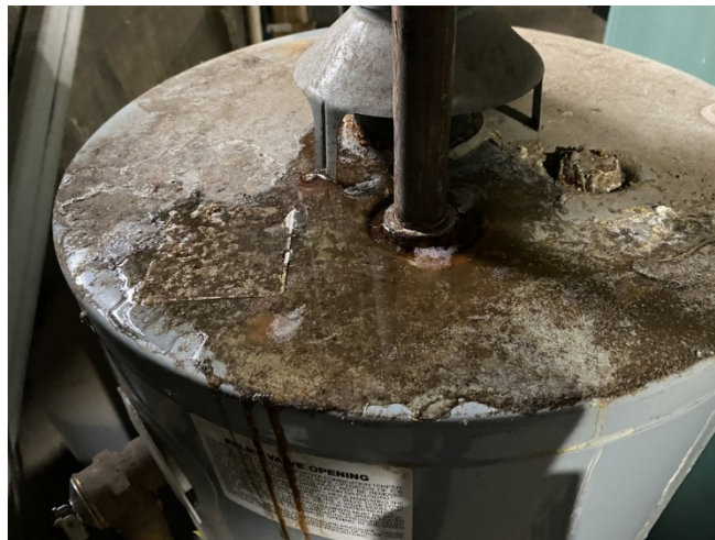
Figure 6: Existing water heater, appears older and may need replacement
