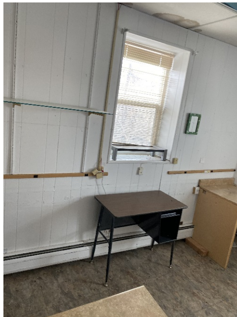
Figure 2: Evidence of water damage
