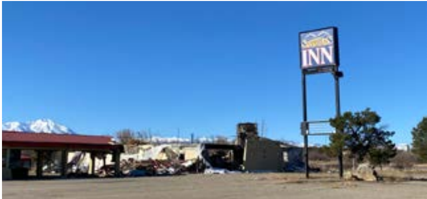
Fire damage on motel and pool house
