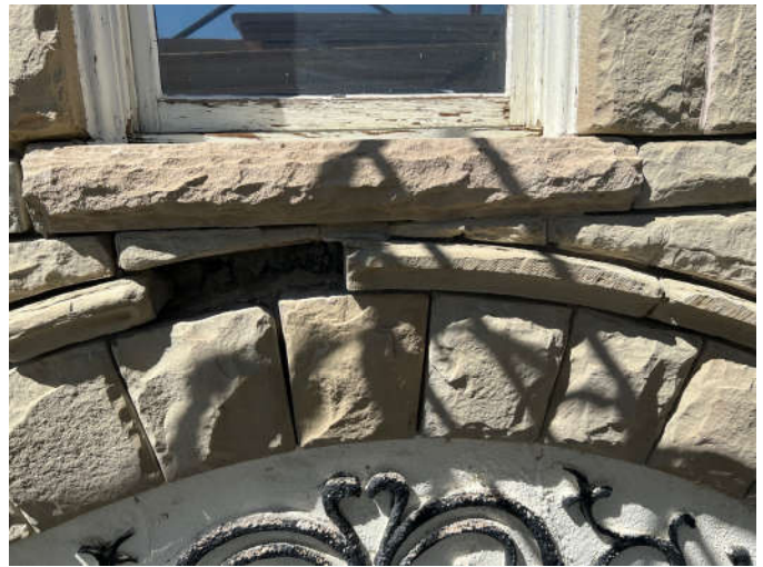
Photo #4: The decorative stone moulding and the small stones below the window sill are eroded. They will be replaced.
