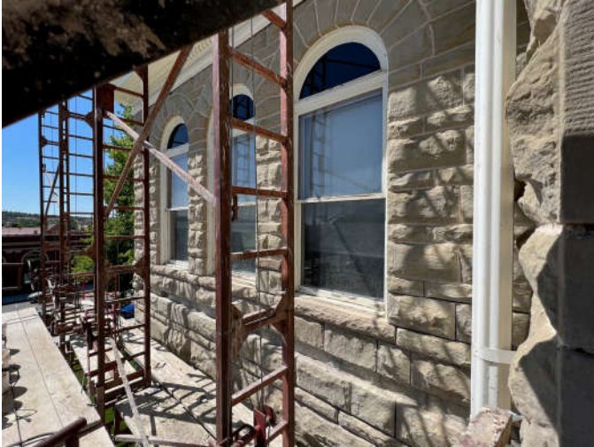
Photo #5: Most of the existing stones that form the projecting string course below the second floor windows have been removed. They will be replaced in-kind.
