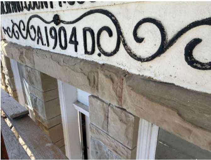
Photo #3: This course of stone, which includes lintels above the window and door openings on the tower's second floor, will be retooled rather than refaced to avoid damage to the plaster sign.
