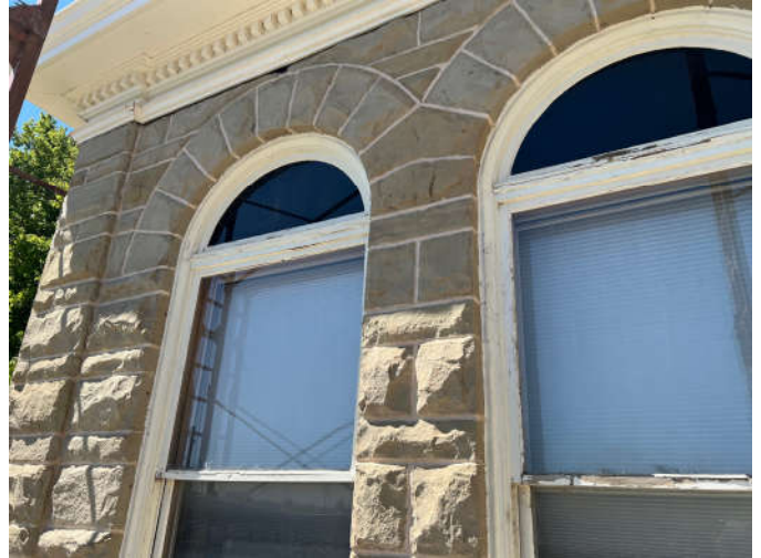
Photo #6: Repointing of the mortar joints is underway, with most joints repointed from the top of the walls to the second floor window sills.
