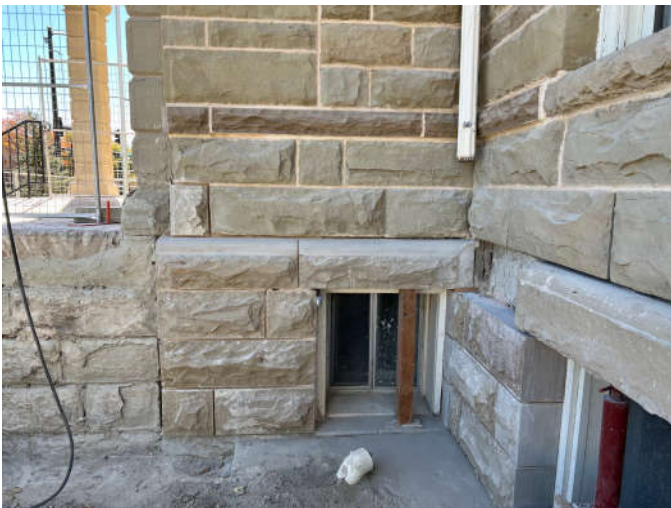
Photo #1: The stones at the bottom of the north tower wall have been replaced. Remaining required effort includes retooling the radiused water table stones and repointing.
