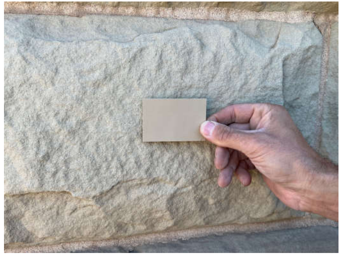
Photo #4: The sheet metal flashing required at the second floor balcony will closely match the color of the stone.
