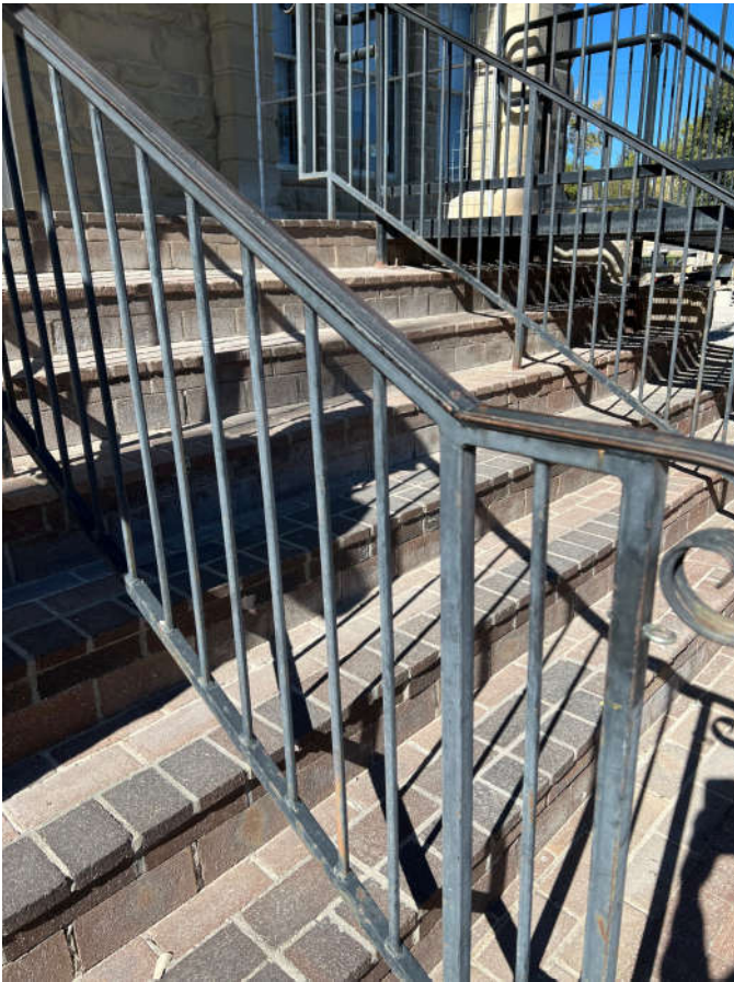
Photo #7: Guardrails are needed along the north and south sides of the main entry porch. Their design should match the existing railing system.
