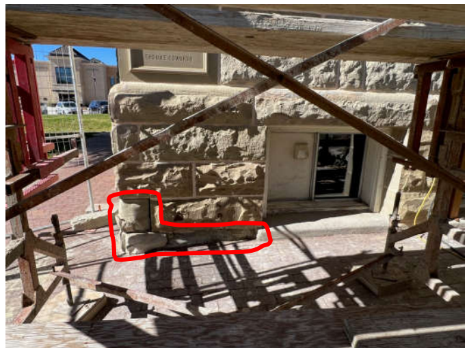
Photo #6: The stones at the bottom of the southeast corner still require replacement. The water table stones above the garden level windows are in poor condition.
