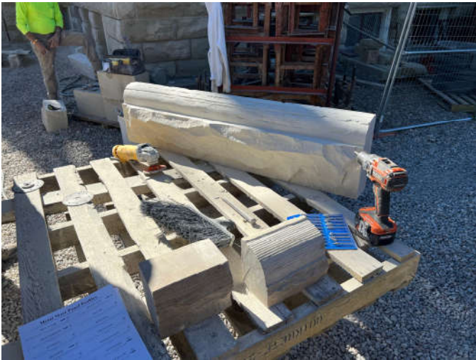
Photo #3: The process for achieving tool marks similar to the original on the radiused top surface of this stone is being tested here.
