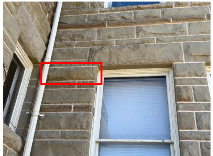
Photo #2: The south bearing stone at this window will receive a deep reface. No pinning is required. However, the lintel stone should be shored prior to refacing.
