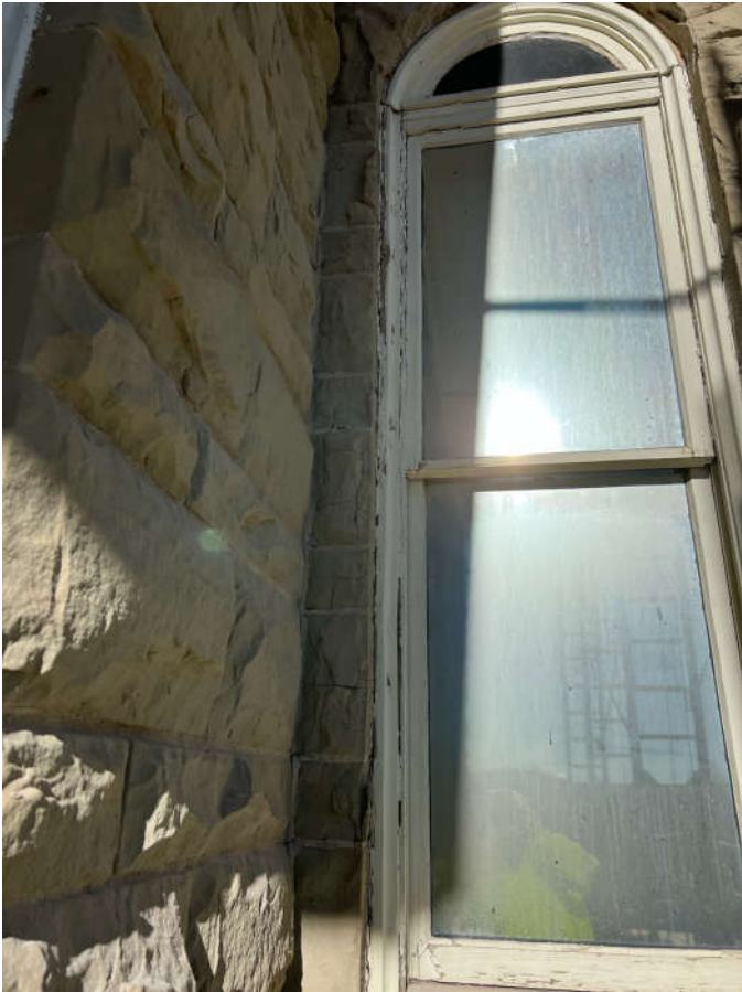
Photo #7: The stones on the west jamb require replacement. (Photo by Mountain Masonry)
