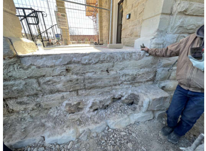
Photo #4: West end of north cheek wall. Some of the non-original stones have not yet been removed.
