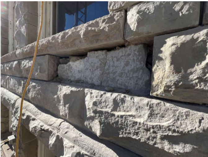
Photo #5: The stone at this location at the south side of the east wall was specified to be refaced.
