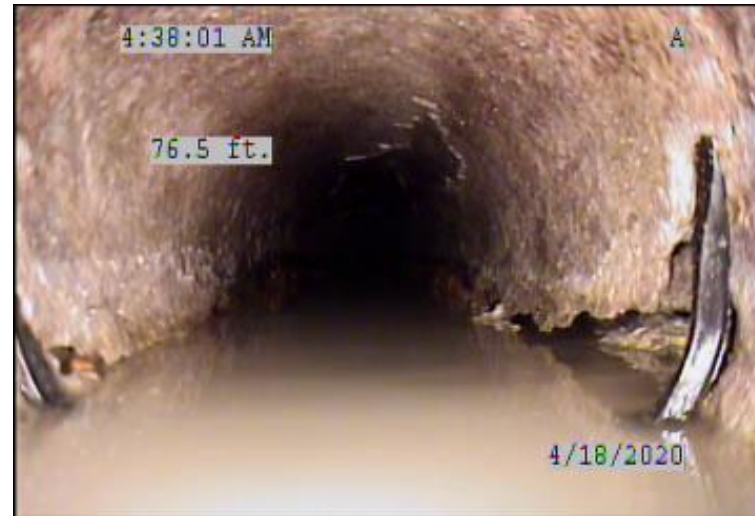
Photo 62: Structural damage (pipe deterioration) (Basin E4).
