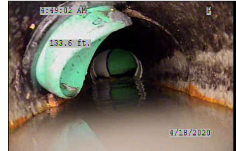
Photo 63: Protruding lateral (Basin E4).
