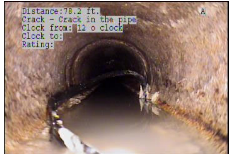
Photo 61: Structural damage (crack in pipe) (Basin E4).
