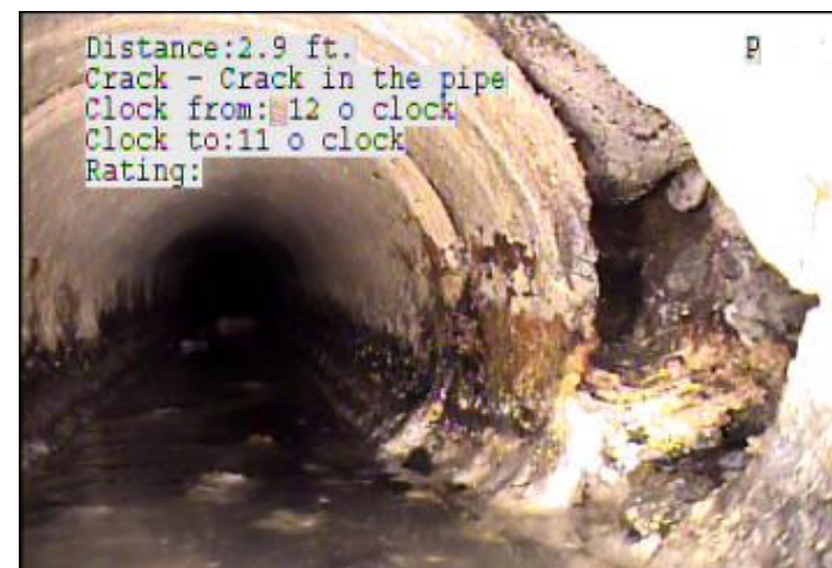
Photo 65: Structural damage (hole in pipe) (Basin E4).
