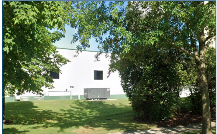
Homewood Flossmoor Generator
