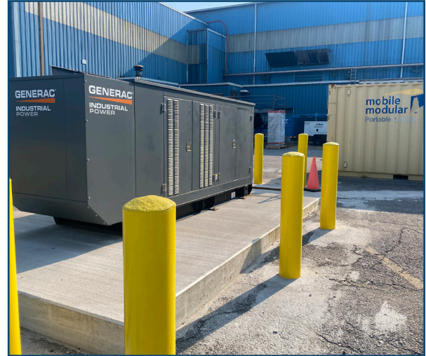
New Backup Electrical Generator Installed for NMLK Indiana
