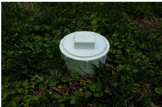
PVC Sewer Cleanout
