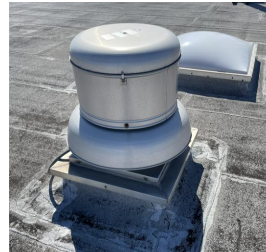
Typical roof mounted exhaust fan
