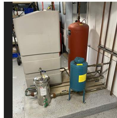
Police Station ground loop equipment (glycol feeder, expansion tank, pot feeder & side-stream filter)
