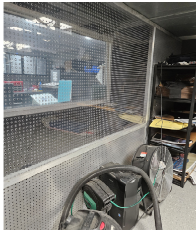
Shooting Range perforated supply air wall
