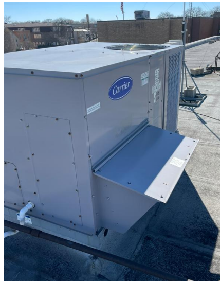
Fire Station dormitory rooftop unit
