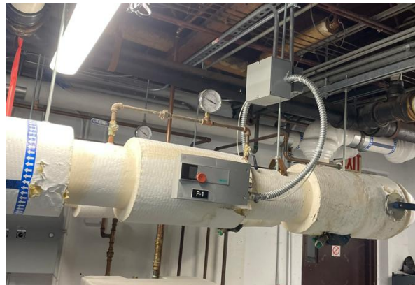
Police Department ground loop pumps
