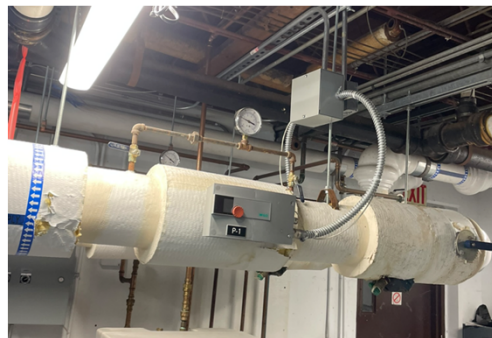
Police Department ground loop pumps
