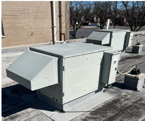
Police Department energy recovery ventilators
