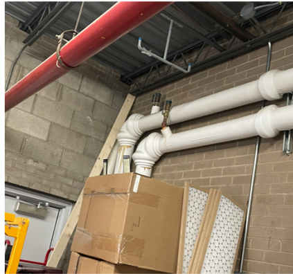
Piping to / from geothermal field (Police Department)
