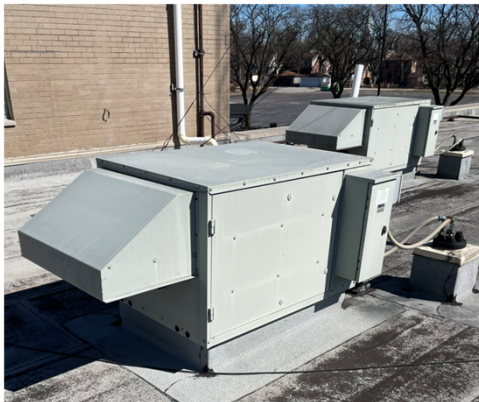
Police Department energy recovery ventilators
