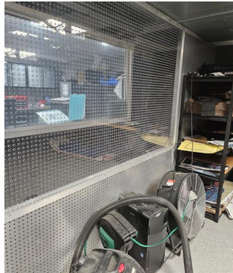
Shooting Range perforated supply air wall
