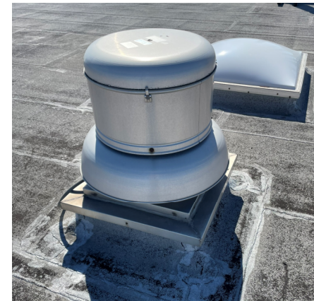
Typical roof mounted exhaust fan
