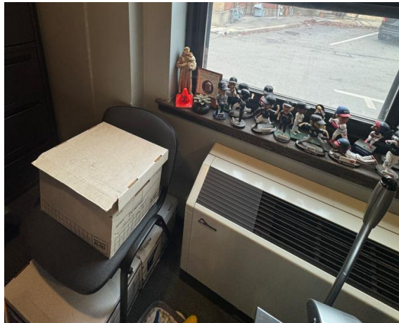
Typical floor-mounted HP
