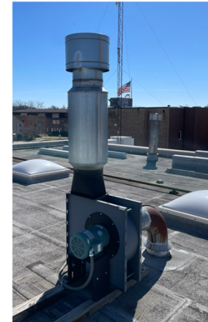
Apparatus Bay source-capture exhaust fan
