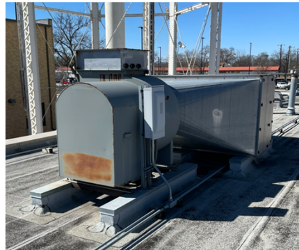
Shooting Range exhaust fan and HEPA filter housing
