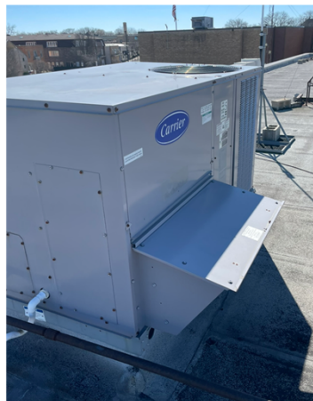
Fire Station dormitory rooftop unit
