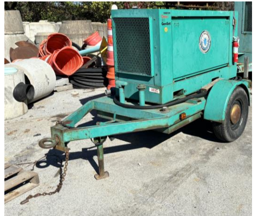
Old 1984 ONAN 30kw towable generator
