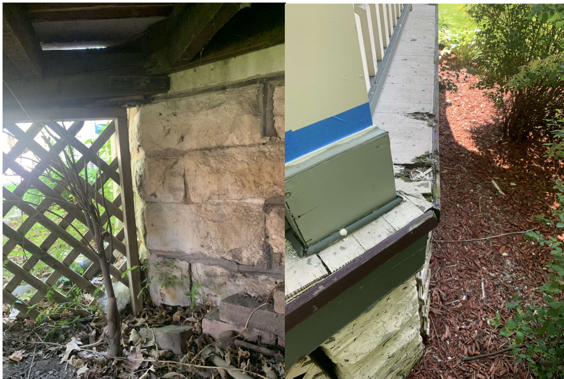
EXAMPLES OF ROTTING WOOD ELEMENTS
