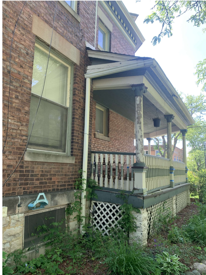
VIEW OF SIDE OF PORCH & SLIPPAGE
