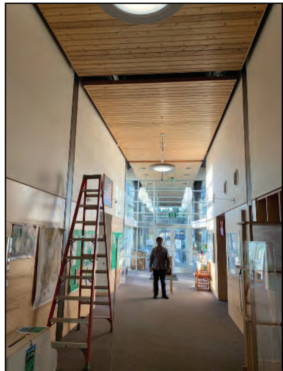
Structural frame for a security gate that was built in to the Library's entry hall.
