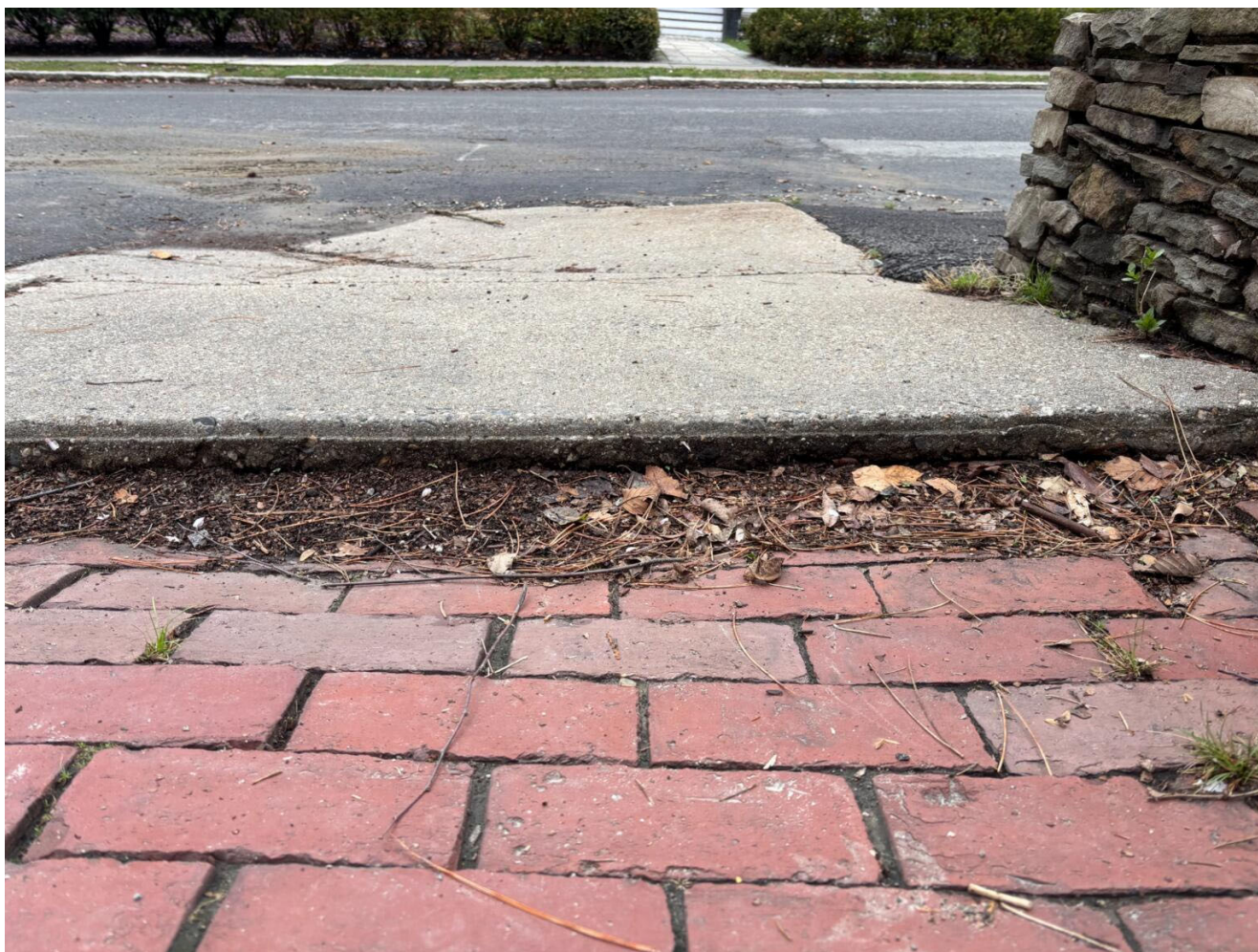
A close-up of an unsafe sidewalk transition in the author's neighborhood. (Courtesy Barbara Thimm)
