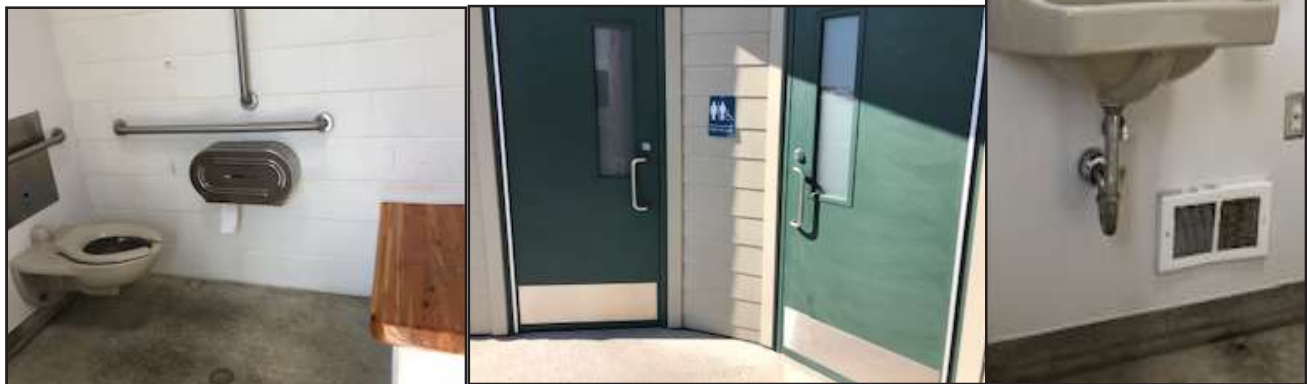
This project will correct accessibility issues at City of Homer public restrooms. Some depicted here include improperly placed dispensers and grab bars, lack of wheel chair space from bench, incorrect door swing and lack of cover on the lower pipes
