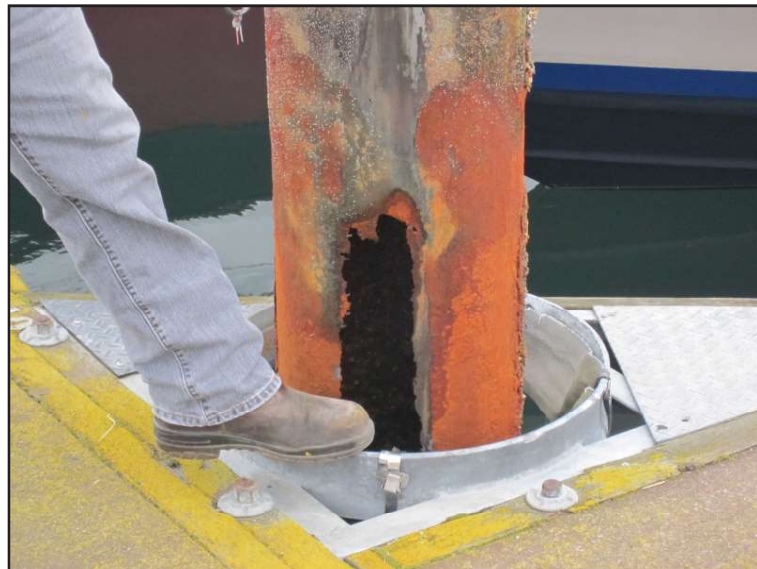
Example of the damage electrolysis causes to harbor pilings. This broken piling in 2012 caused the R & S floats in the harbor to be condemned until it could be repaired.
