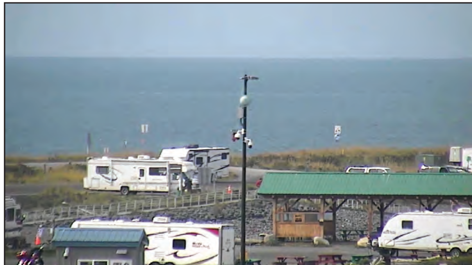
Security cameras, pictured here, center, allow harbor officers to gain situational awareness before responding to an event, to verify details of recorded events and monitor progress of evacuations or check on inundation during tsunami events.
