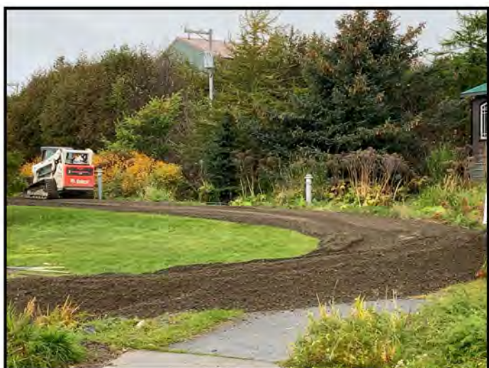
Contractors improved the surface of the Story Trail at Homer Public Library with new fabric and surface material.
