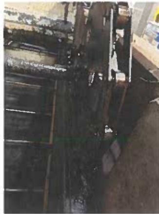
Figure 2: Clarifier 2 Southeast Sprocket and Damaged Drive Chain
