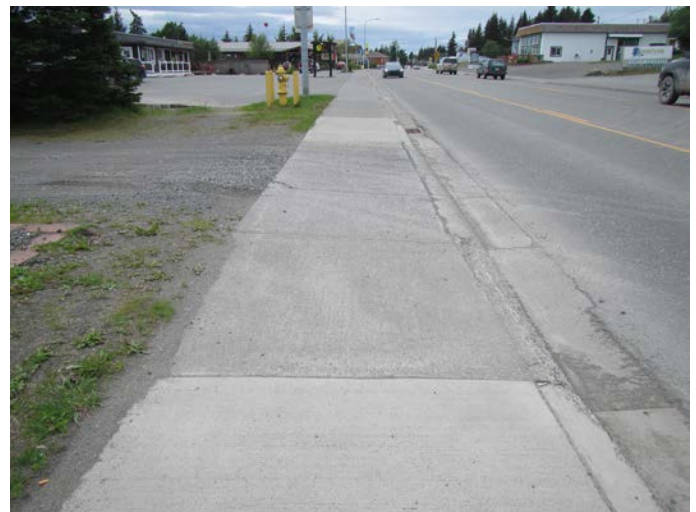
Figure 20: Driveway Entrance with Steep Cross Slope
