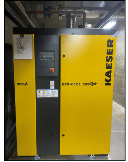
New Kaeser blower unit
