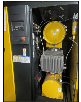
Control panel and inside mechanisms
