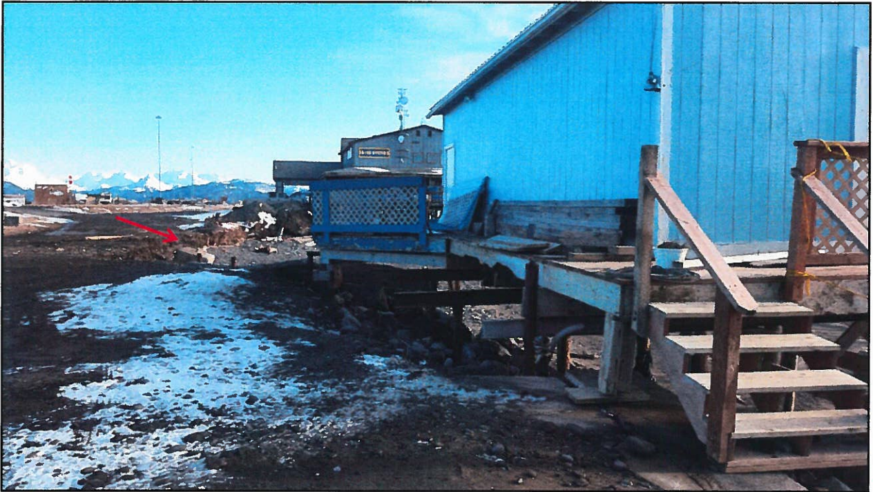
View SE from close to the parcel's north boundary. Photo was taken from near the middle of the "lot". Washing-out under the improvements has become worse in recent years. Lessee is in the process of doing major site work to try and further stabilize the erosion cutting in underneath the improvements. Eroded area at arrow is within the State R-O-W.
