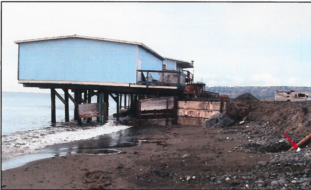
Close up view from midway on the eastern undeveloped portion of the site (see survey). The exposed sewer line is noted at arrow.
