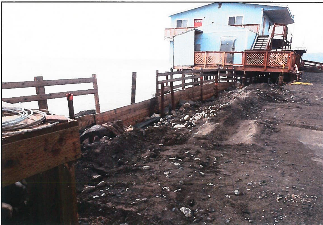
Close-up view to work in progress in front of the seawall between the two buildings.
