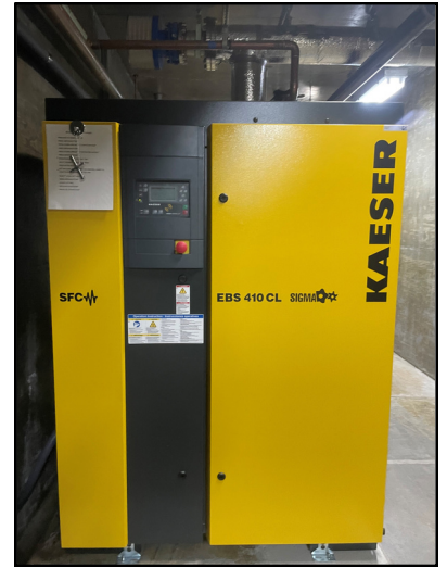
New Kaeser blower unit
