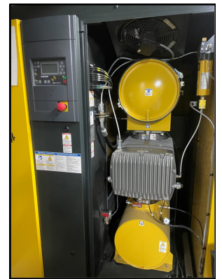
Control panel and inside mechanisms
