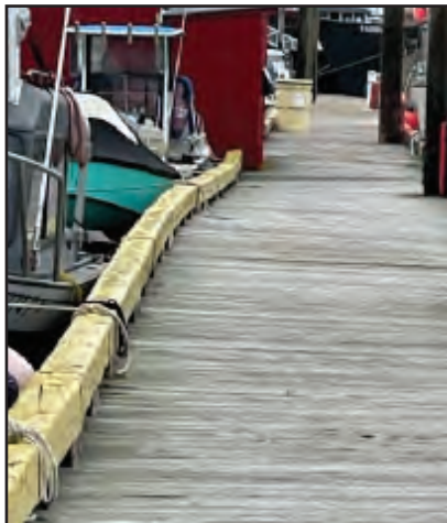
The Headwalk Float AAA is warped, suggesting a failure in the structural members below the deck and lack of flotation..
