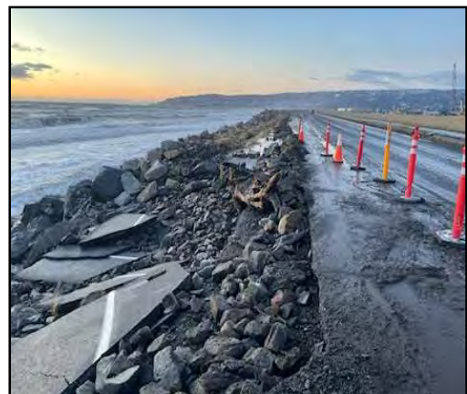
2024 erosion damage triggering disaster declarations.
