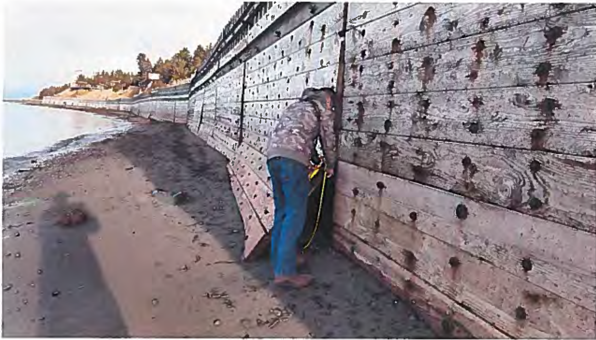
Figure 5 - HDR, Inc. inspection of wall to assess damage in support of recommending potential long term improvements
