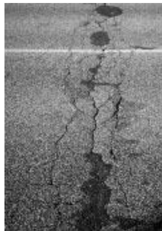
▲ Water enters unsealed cracks softening pavement and forming secondary cracks.
