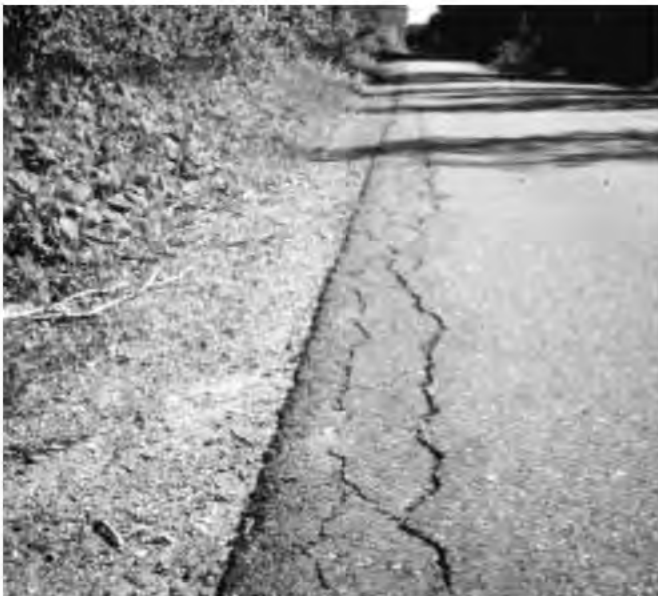
Highshoulder and no ditch lead to pavement damage. Needs major ditch improvement for a short distance. RATING: Fair
