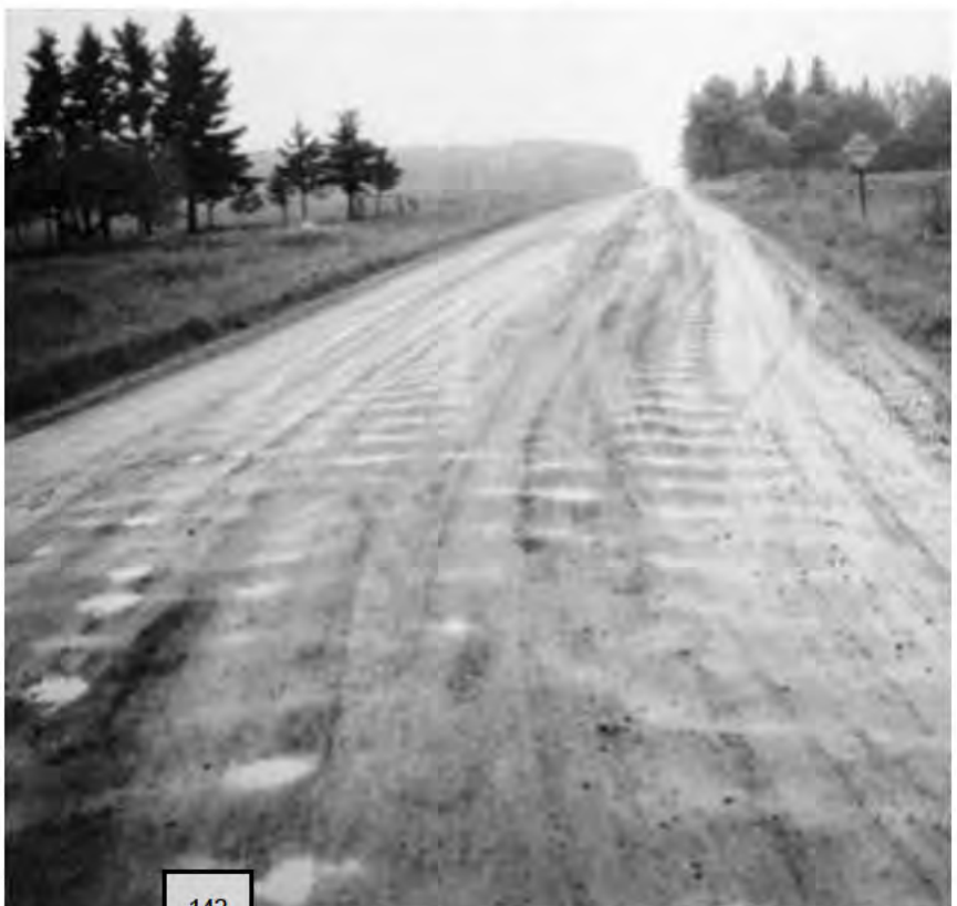
► Severe washboarding traps water.
