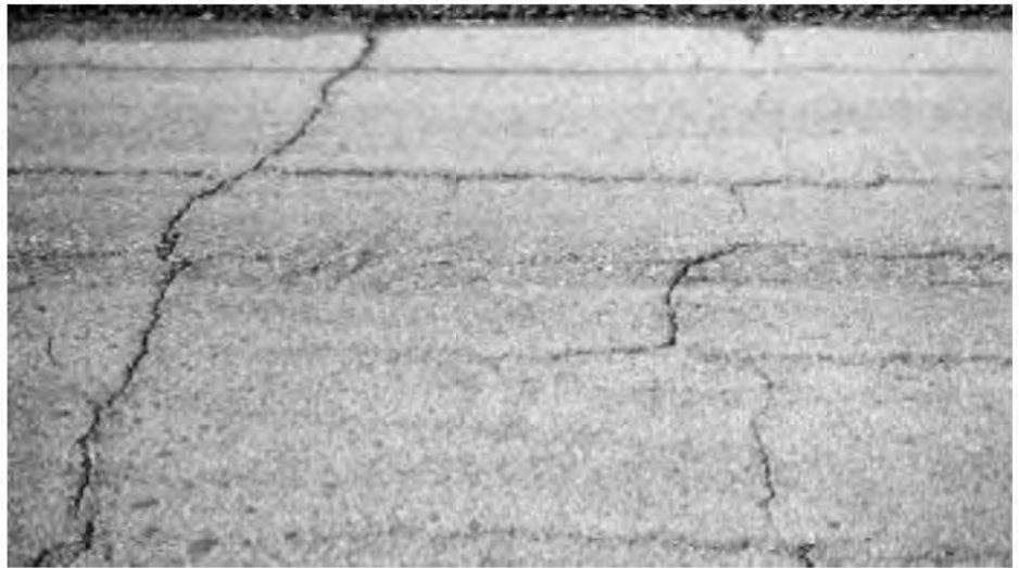
▼ Block cracking with open cracks.
