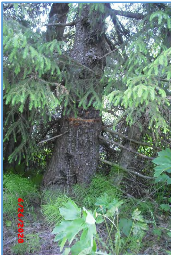
Figure 7: Tree, well inside right of way, scarred from grader during snow removal
