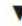
Partial drainage. Ditch and new culvert being added on left. Little or no drainage on right.
