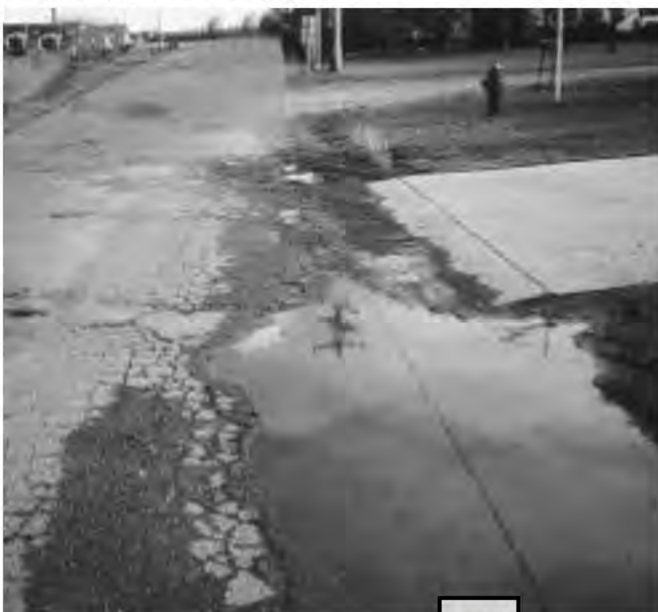
No drainage leads to failed pavement. RATING: Poor
