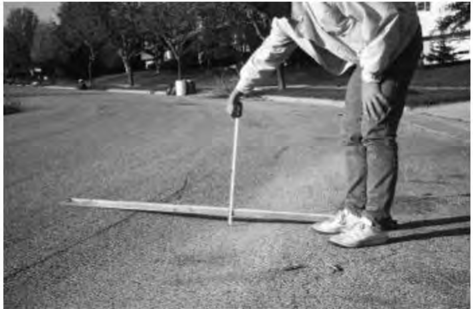
► Severe settling from utility trench.
