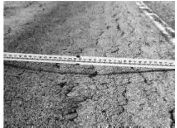
▲ Severe rutting. Strengthen base and reconstruct.
