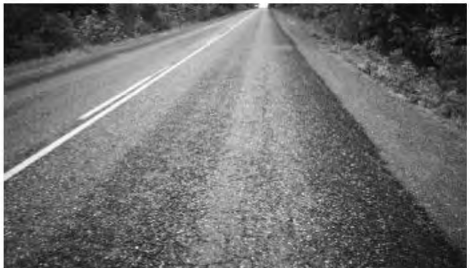
► Moderate to severe raveling in wheel paths.
