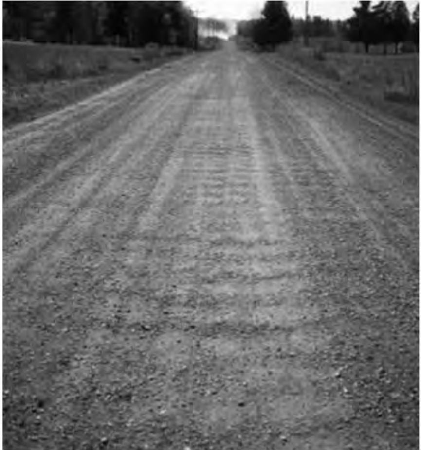
▼ Moderate washboarding in center of road.
