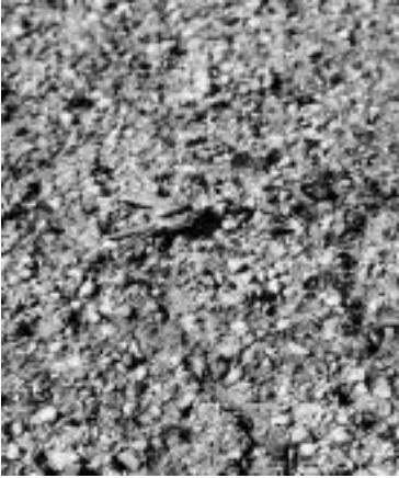
Severe raveling with ▼ extreme loss of aggregate.
