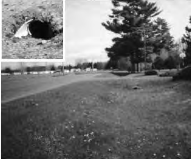
Good rural ditch and driveway culvert. Culvert end needs cleaning. RATING: Good
