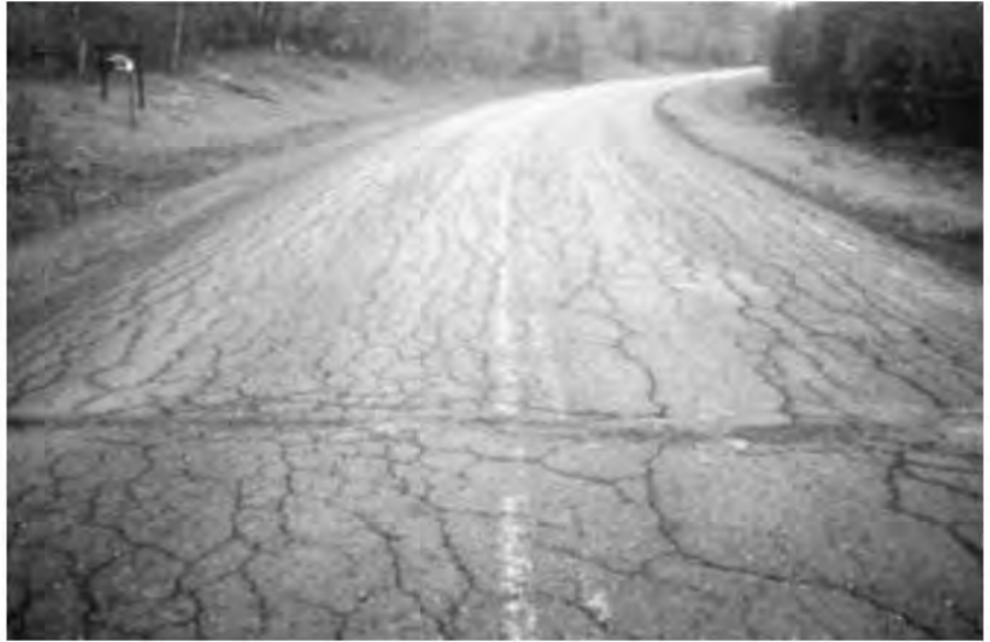
▶ Extensive alligator cracking. Pulverize and rebuild.
