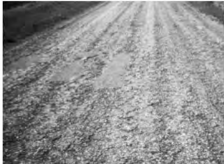
◀ Severe raveling and loss of surface material.
