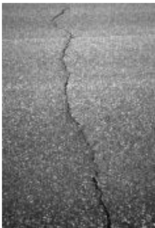
▲ Tight cracks less than 1/4" in width.
