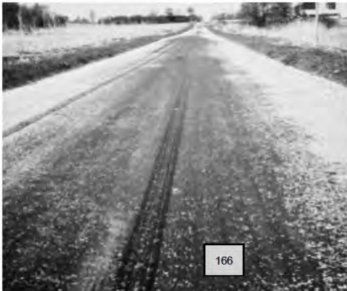
► Flushing. Dark patches show where asphalt has worked to surface.
