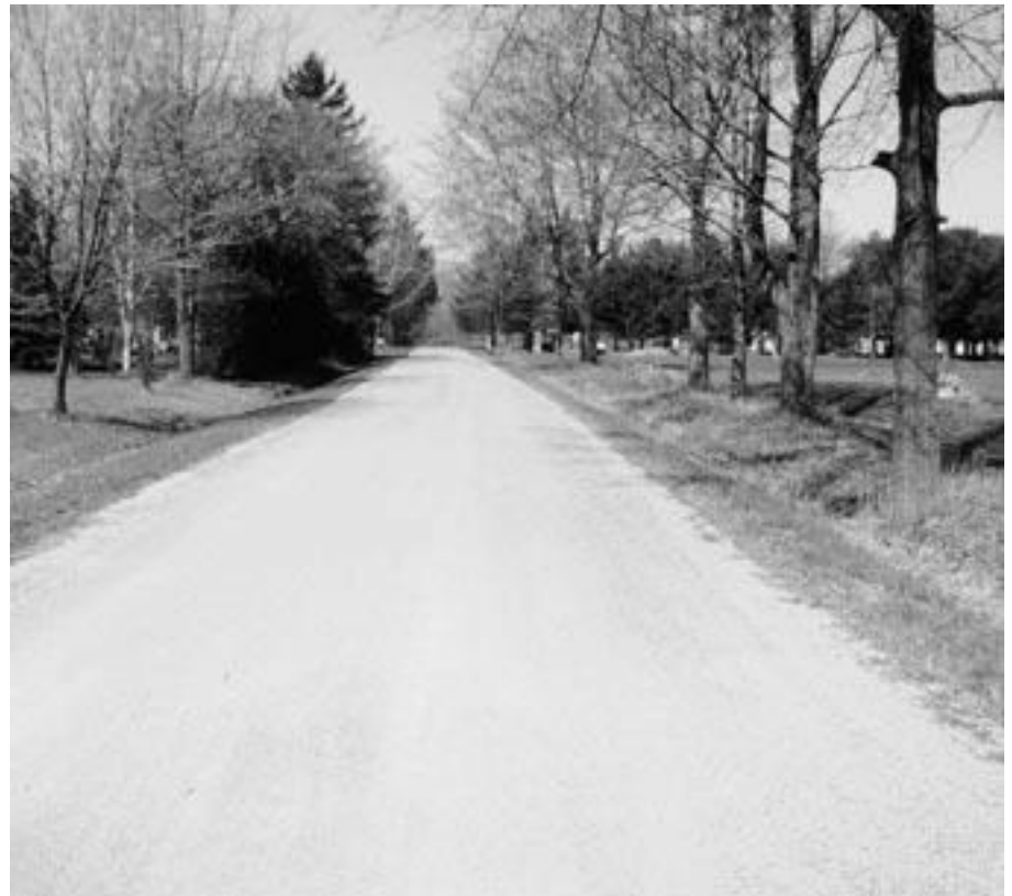
► Road has excellent crown. Gravel has been stabilized for dust control. Very good drainage.
