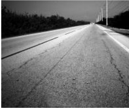
Load cracking and slight ▼ rutting in wheel path.
