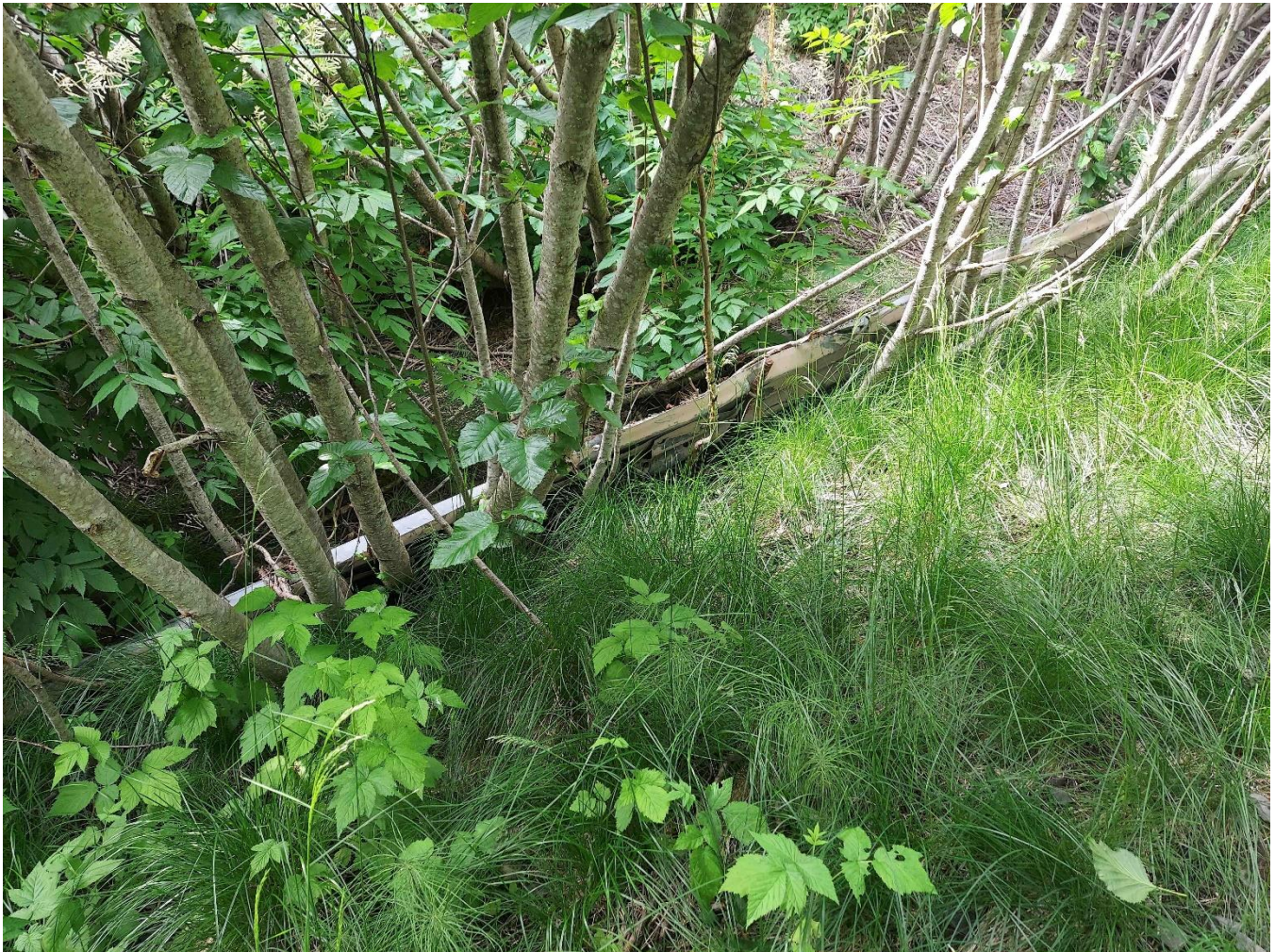
PHOTO 2: The photo above shows the same retaining wall shown in the previous photo that has been tipped over (leaning away from the slope) by the sloughing hillside and partially buried as well.
