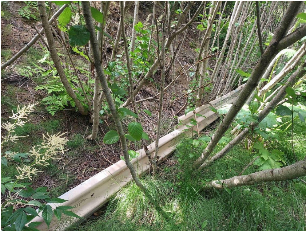
PHOTO 1: There are several locations where rebar was pounded into the soil and “roadway guardrail” was used at the toe of the upgradient cut slope along the roadway going up the hill to retain the slumping hillside from falling onto the road. This is not a generally accepted method of constructing a retaining wall (materials used or construction method).
