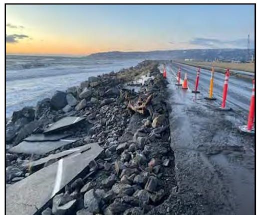
2024 erosion damage triggering disaster declarations.
