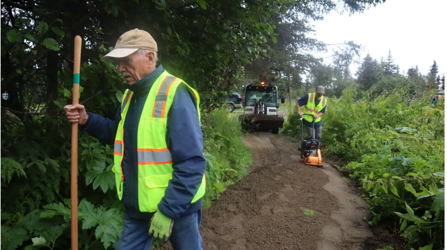
Volunteer Mike Haines raking gravel while Parks Coordinator Chad Felice operates the Toolcat and Parks Technician Matt Hornaday runs the compactor on the upper section of Calhoun Trail.
