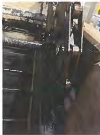
Figure 2: Clarifier 2 Southeast Sprocket and Damaged Drive Chain
