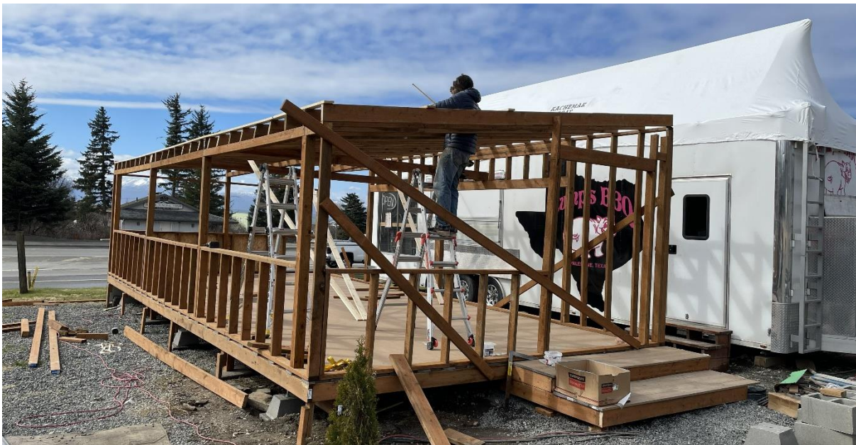
Unpermitted construction located at 3582 Main St. (5.6.26)
