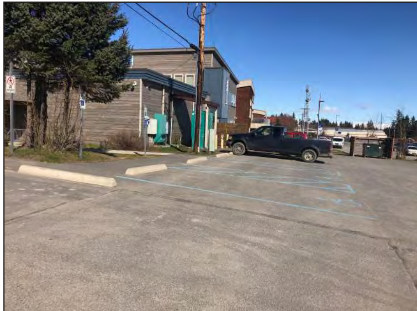
The cross slope of the accessible parking spaces at the lower entrance to City Hall exceeds the maximum allowed 1:48 under ADA standards.
