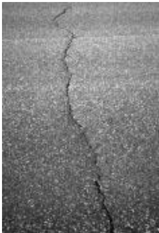
▲ Tight cracks less than 1/4" in width.
