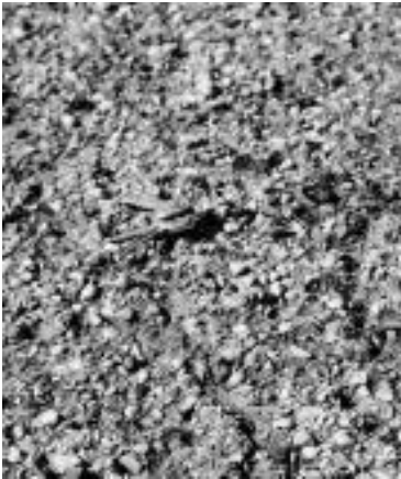
Severe raveling with ▼ extreme loss of aggregate.
