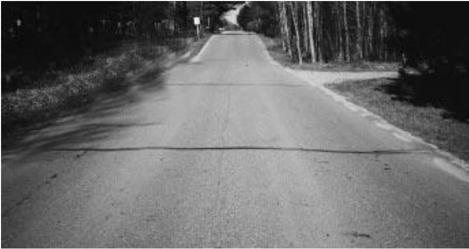
▼ Widely spaced, well-sealed cracks.
