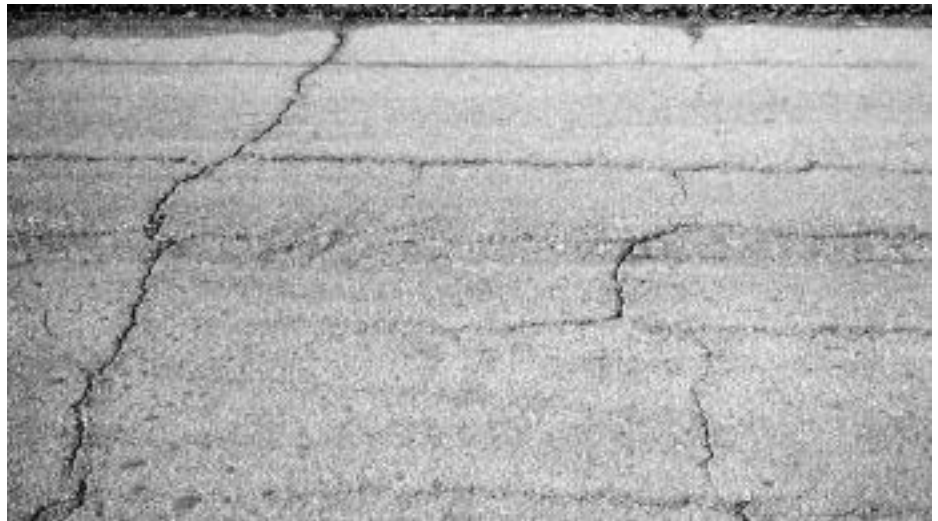
▼ Block cracking with open cracks.
