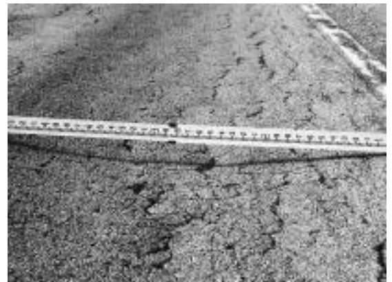
▲ Severe rutting. Strengthen base and reconstruct.
