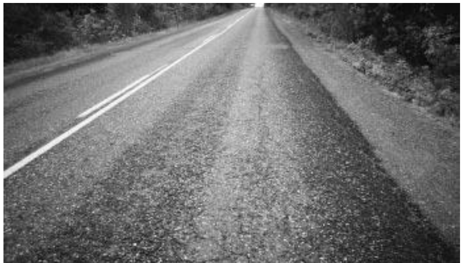
► Moderate to severe raveling in wheel paths.
