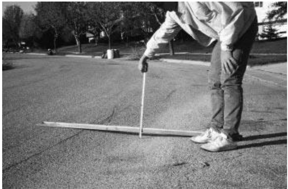
► Severe settling from utility trench.
