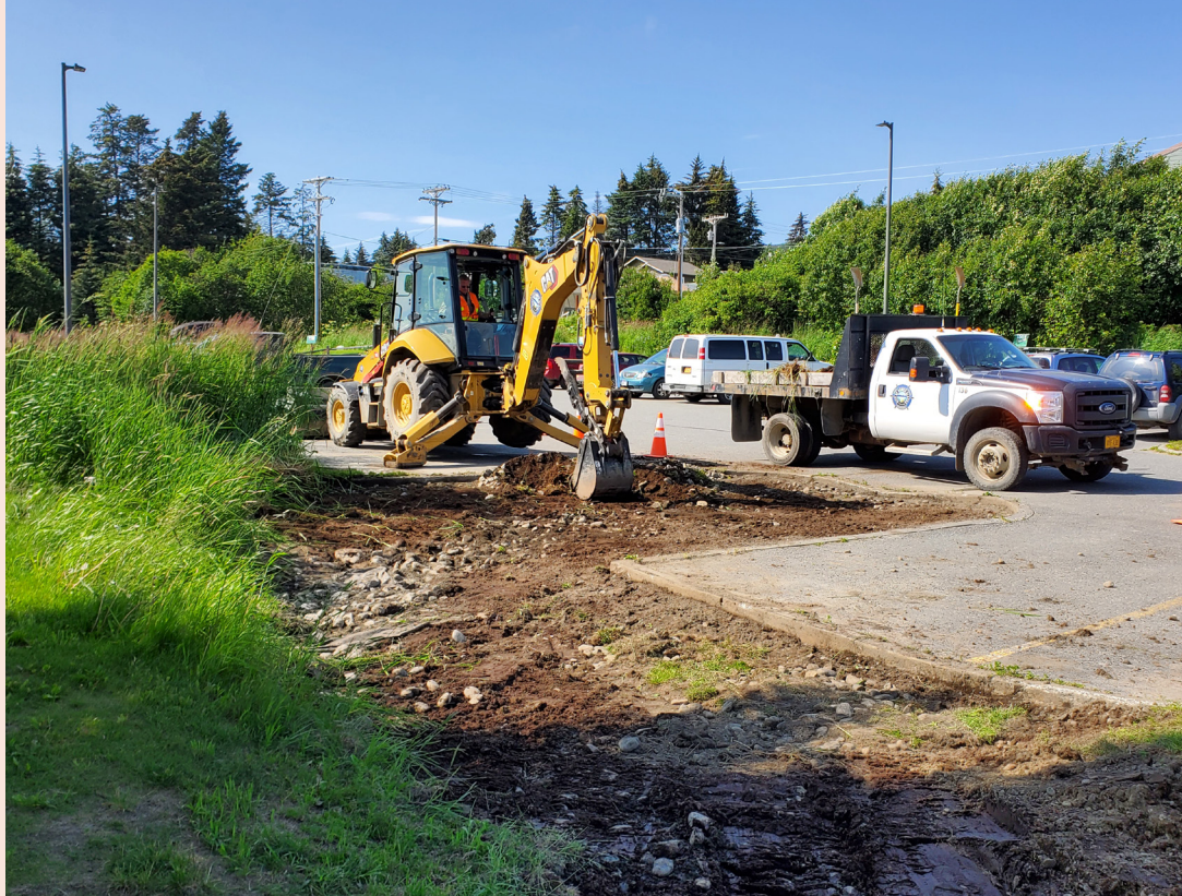
Staff from Public Works dredged out the drainage channel on the south side of the parking lot on August 15
