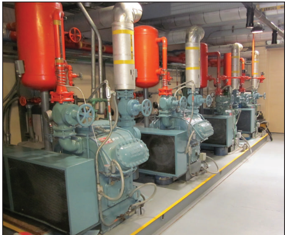
Four of the Ice Plant's aging compressors are shown here.
