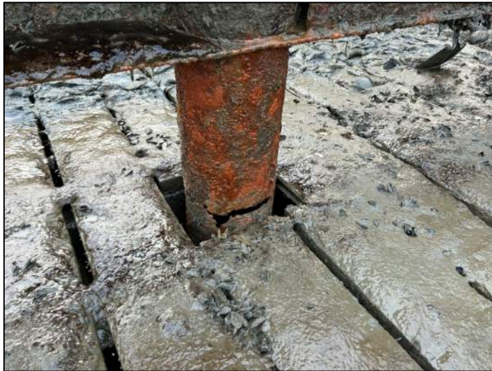
Figure 1-10. Hole in Pile Under Beam 7
