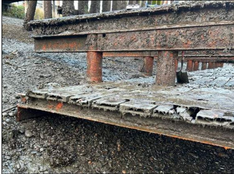
Figure 1-8. Degradation of Wood Decking
