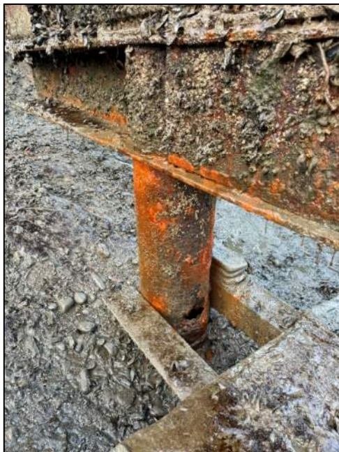
Figure 1-11. Hole in Pile Under Beam 5
