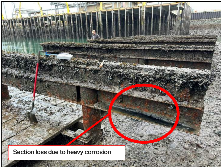
Figure 1-6. Section Loss Due to Corrosion
