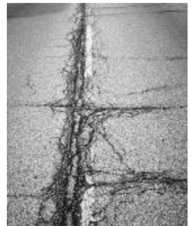
▲ Pavement ravel and erodes along open cracks causing deterioration.
