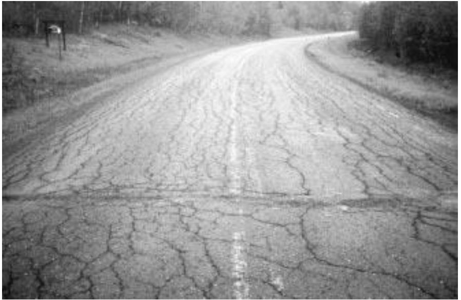
▶ Extensive alligator cracking. Pulverize and rebuild.
