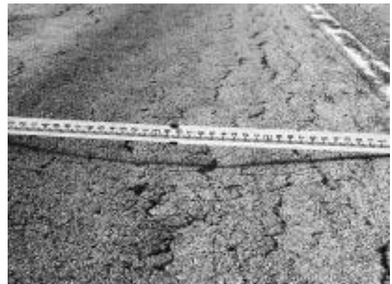
▲ Severe rutting. Strengthen base and reconstruct.
