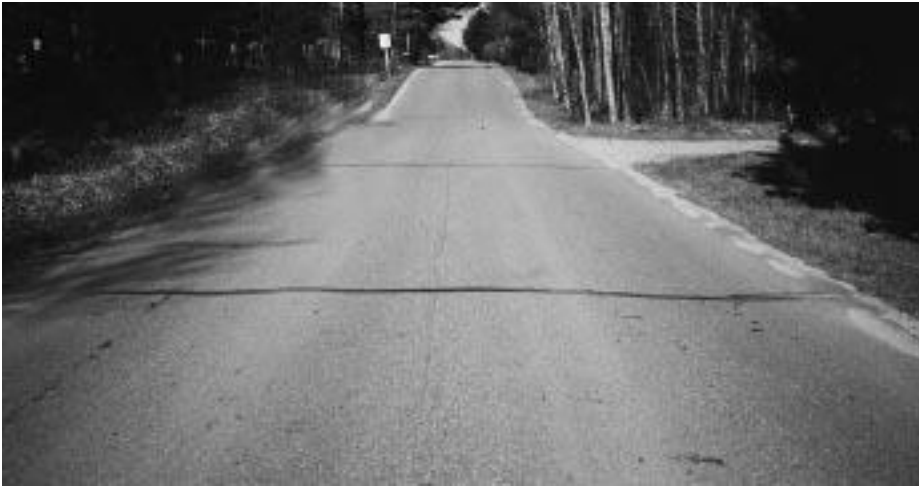
▼ Widely spaced, well-sealed cracks.
