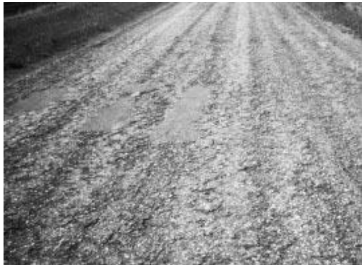
◀ Severe raveling and loss of surface material.
