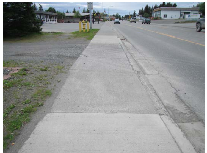
Figure 20: Driveway Entrance with Steep Cross Slope
