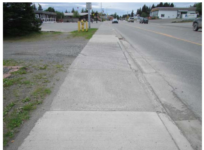
Figure 20: Driveway Entrance with Steep Cross Slope
