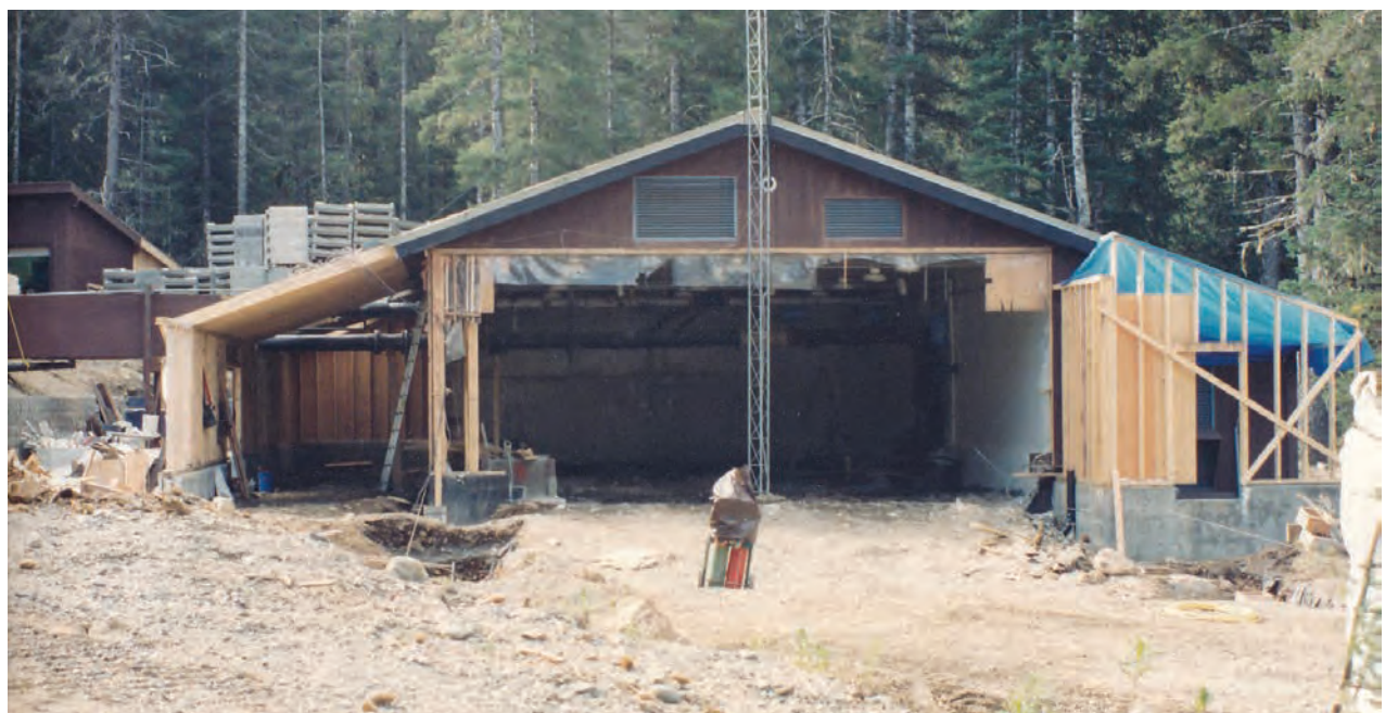
Tutka Bay Lagoon Hatchery under construction to expand the size. This expansion took place when CIAA acquired the hatchery from the State of Alaska in 1991.
