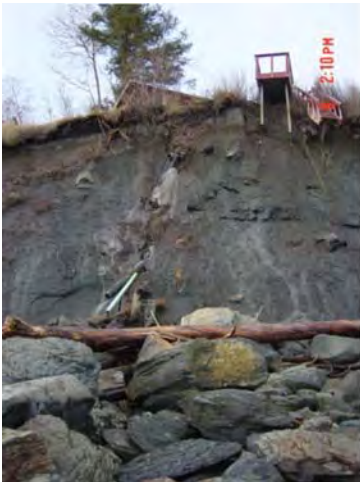
Photo 2: Homer Bluff erosion December 2006
