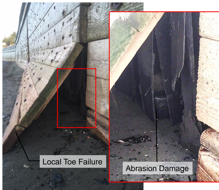
Figure 4. Example of observed local failure – correlates to sink hole at top of the seawall. Inset shows previous assumed abrasion damage.
