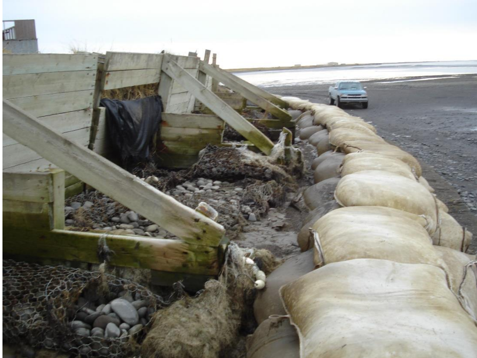
Figure 10. Example of geotextile container revetment (pyramid layout). In the Homer seawall case, the containers would be placed against the seawall.
