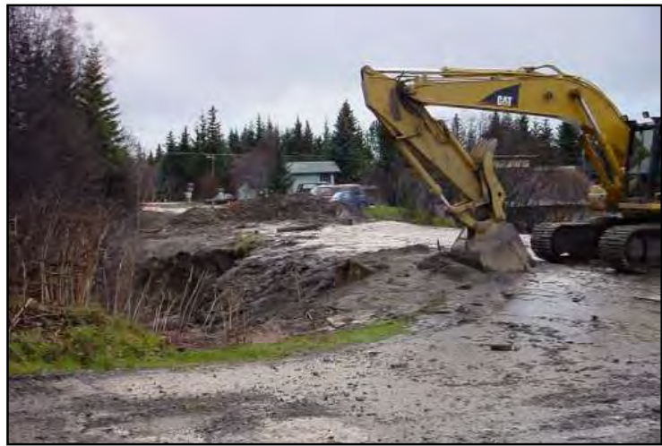
The Slope Stability Program utilizes nature based and low impact development techniques to mitigate erosional damage and protect water quality.
