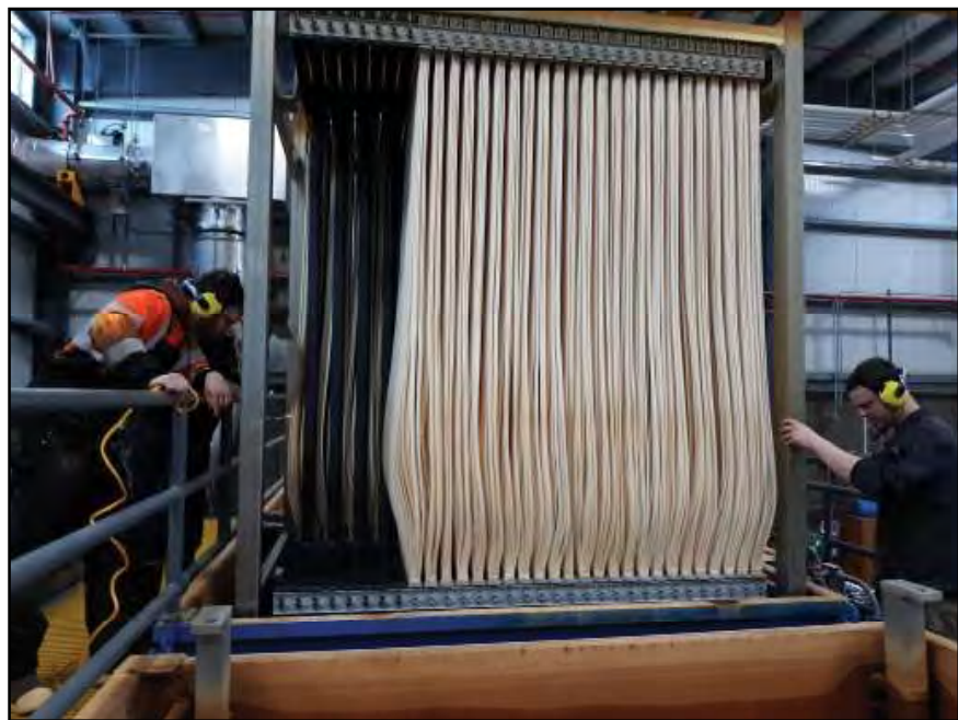
City of Homer Waste Water Treatment Plant staff checking a membrane tray for leaks
