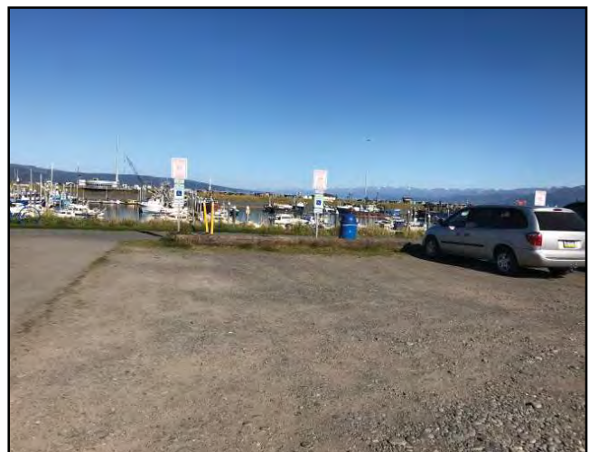
While inaccessibility issues in these Port & Harbor parking spaces have been remedied, it provides an example of spaces needing to be paved with an even path of travel.
