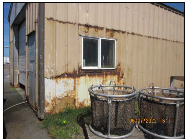
Corrosion is compromising the Fish Grinding building’s structural integrity and degrading interior fixtures.
