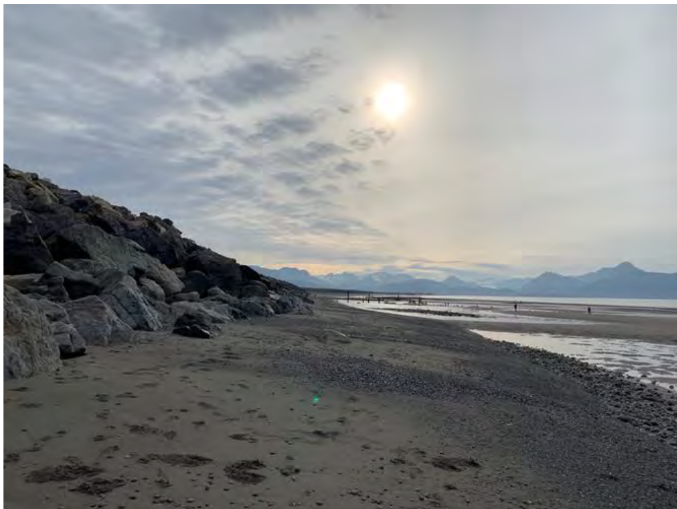
Figure 3. Condition of USACE revetment along the Spit.
